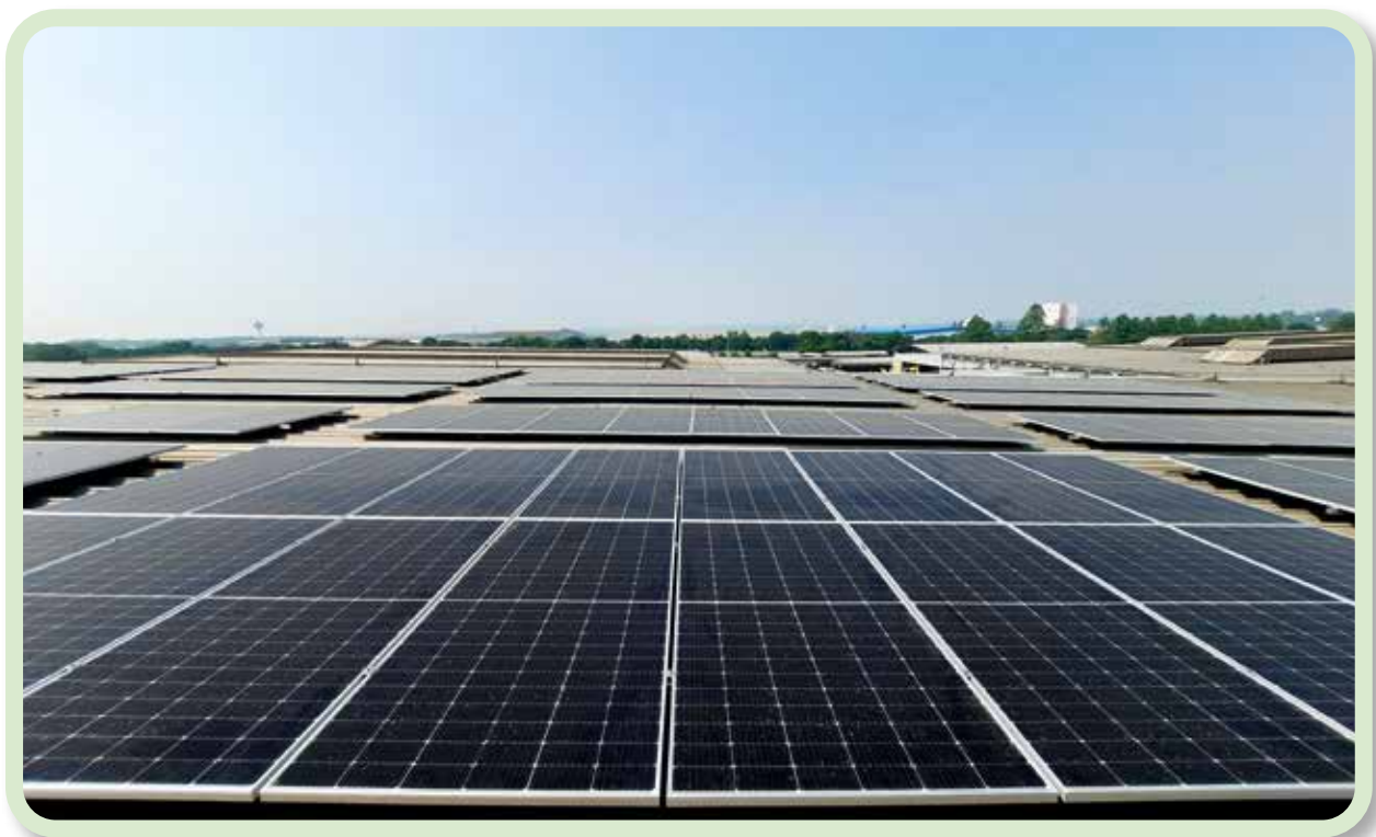
Fasilitas panel surya memanfaatkan Energi Baru Terbarukan (EBT) di Pabrik-1 Karawang Solar panel facility utilising New Renewable Energy (EBT) at Plant-1 Karawang
